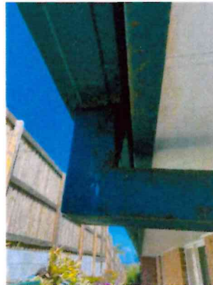
This downpipe on the NE corner of the garage is badly rusted and leaking. Persistent leaks are a conducive condition for termites.
